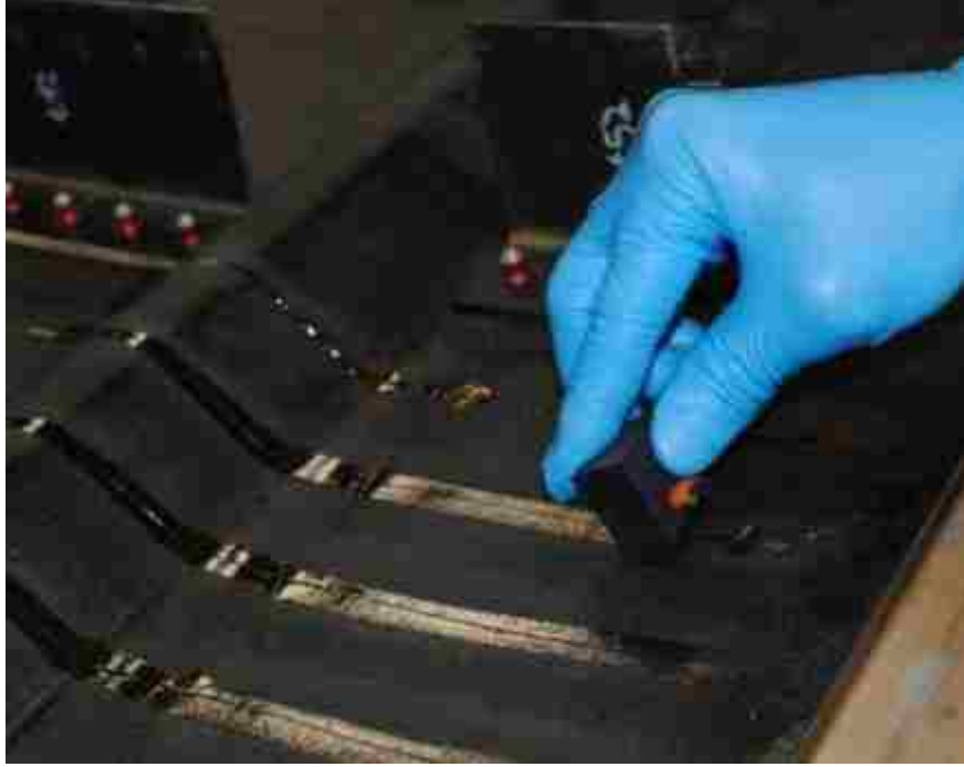
Figure 3-14: Thin Line of M-Bond GA-2 Adhesive Being Squeegeed Smooth Around Fiber Optic
