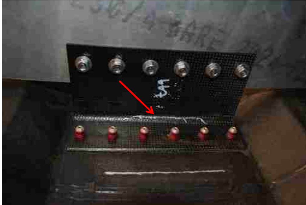
Figure 4-16: Crack on Shear Tie Bend Radius Not Detectable Using NDI from Front Side of Panel
